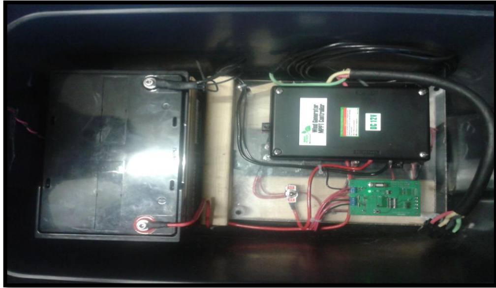
Figure 2 - Inside the P12401 Enclosure
