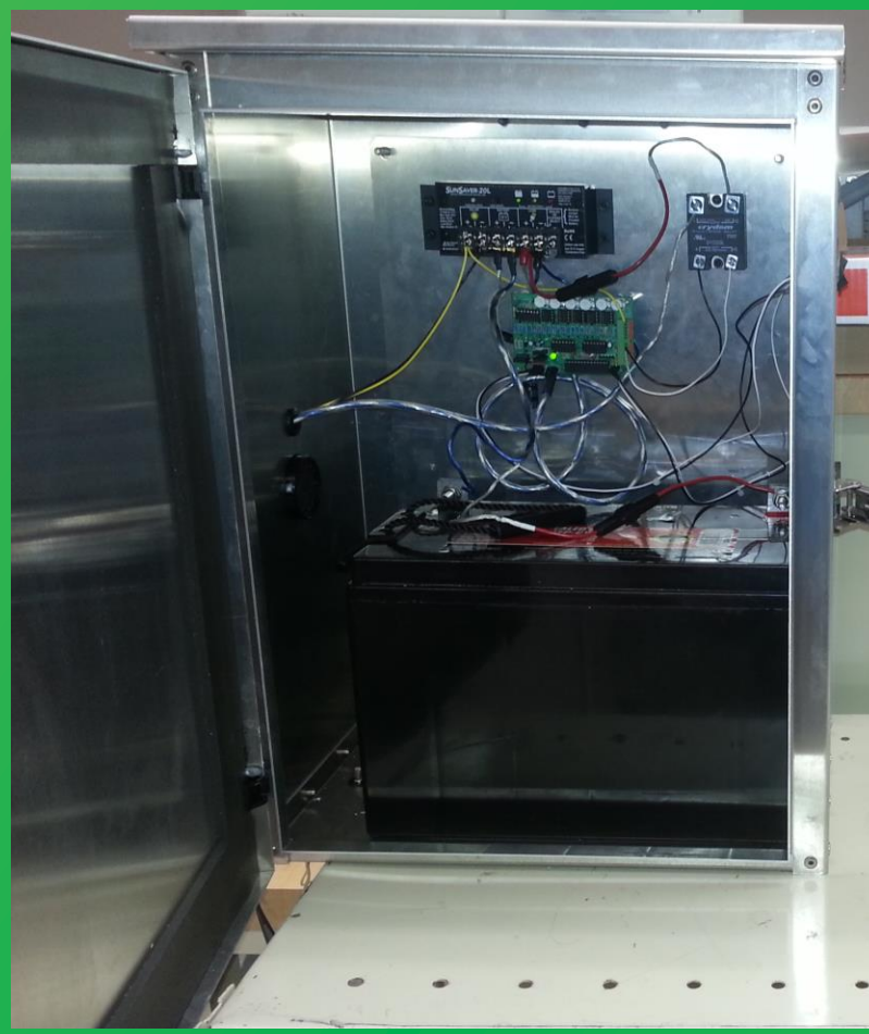
Subsystems within Enclosure
